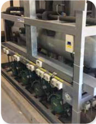
Low temperature CO 2 rack unit
