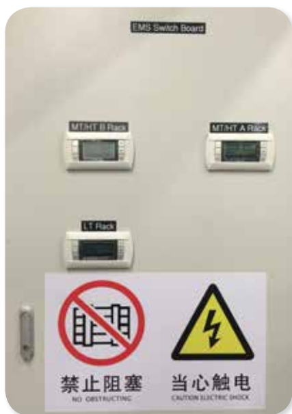
Electrical switch board control
